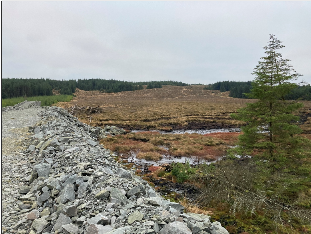
View of head of peat failure along access road to T7 and stabilising berm
